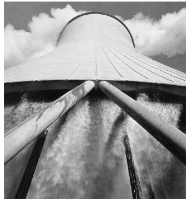
Wet cooling tower
